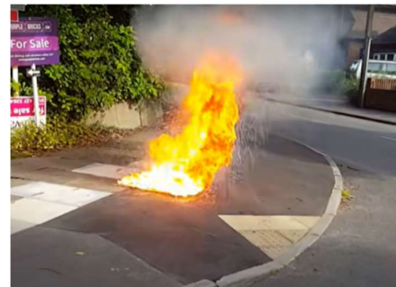
Figure 2. Underground arc fault from an LV pit in the UK [17] (video at 0:36)
