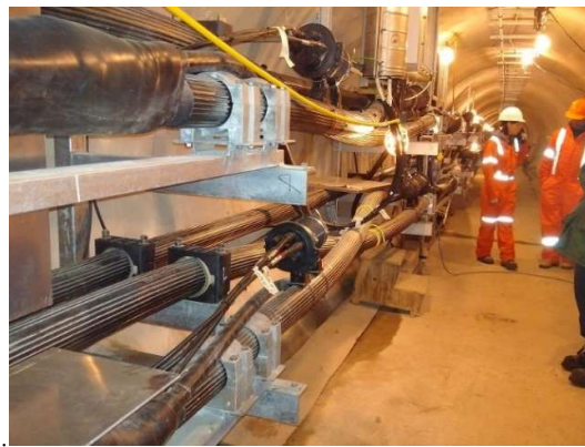
Figure 7. 230 kV Joints in a tunnel showing the location of joints at chest and face level indicating the risk to workers should such a joint fail causing an explosion or an arc-flash [7]
