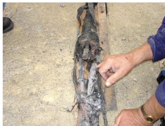
Figure 6. Example of a faulted 33kV oil filled joint with extensive damage from an arcing fault. [7]
