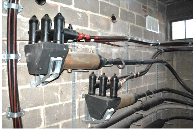
Figure 4. “example of MV PILC/XLPE transition joint containing multiple failure modes of multiple materials: compound filled copper bell, epoxy and EPDM.” [7]
