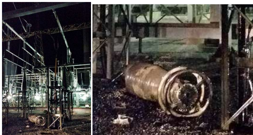
Figure 3. “230 kV Composite Housing Ejected From the Structure” [7]
