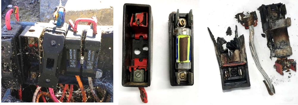
Figure 2 – Example of fuses mounted inside a pillar (left), a fuse base with fuse holder pulled out (middle), a burnt-up fuse base and fuse, with electrical wire with insulation burnt off (right) (Reproduced from –[6])
