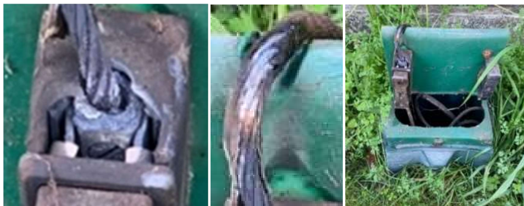
Figure 6 – Signs of pyrolysis (incomplete combustion) such as blackening, soot and brittle of the cable insulation. Also note the damage to the fuse holder and the connector nut and screw. [1]
